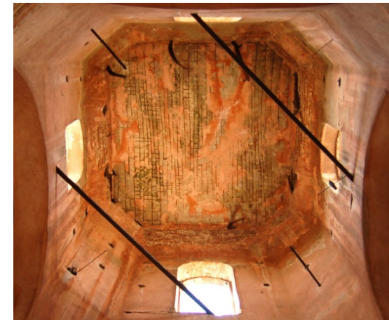
Damages on the upper part of the structure
