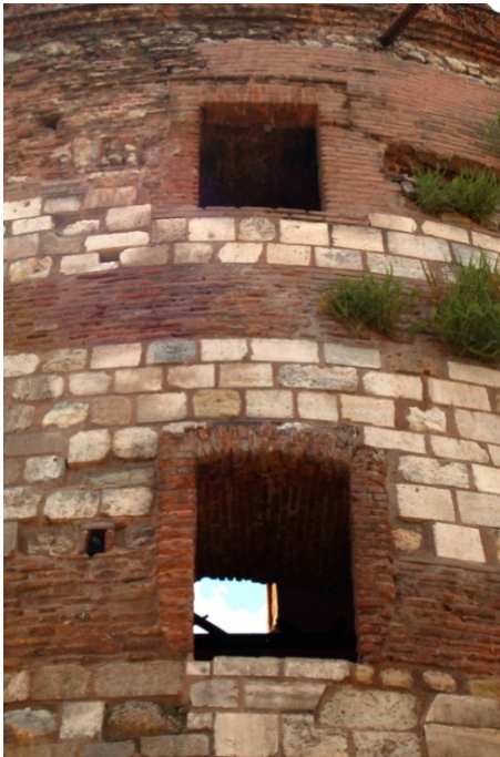
Decay and vegetation on masonry walls
